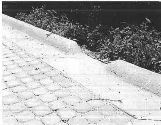
Figure 9.4-B: Cuts in the continuous curb allow for stormwater to be directed into landscaped areas.
